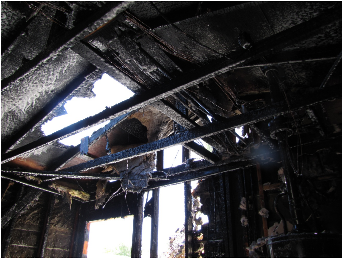
Figure 3: Interior shot of garage showing fire damage to roof and supporting members. This garage had no sheet rock protection of the supporting roof members.
