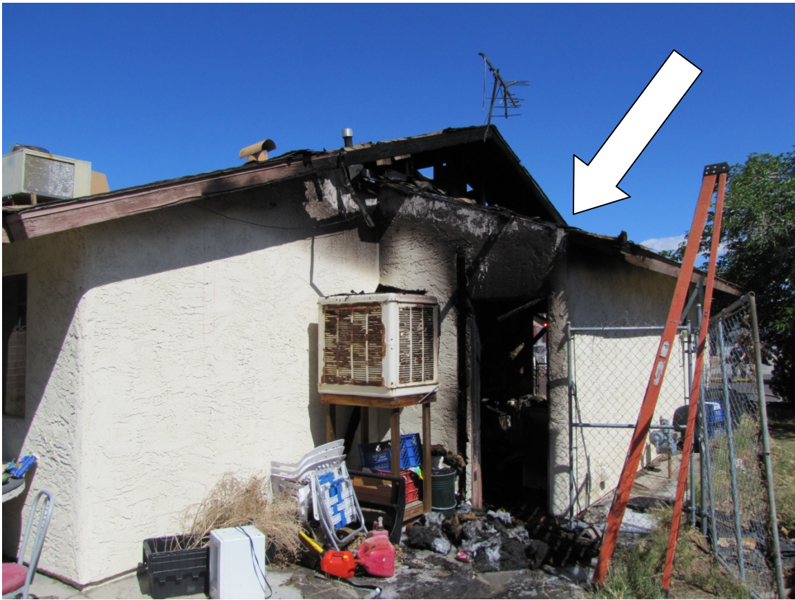
Figure 2: B side of structure showing roof/attic fire damage. Arrow points to area FF fell through on the lower roof.
